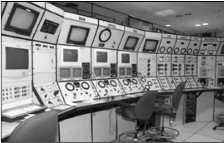
The control panel for the saturation complex at DRDC Toronto is impressive.
